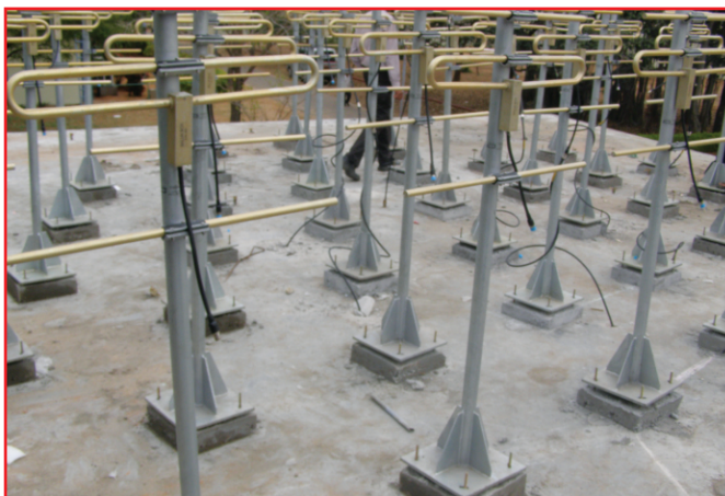
Work is in progress for the mini profiler (49 subarray) at ECIL, Hyderabad.
