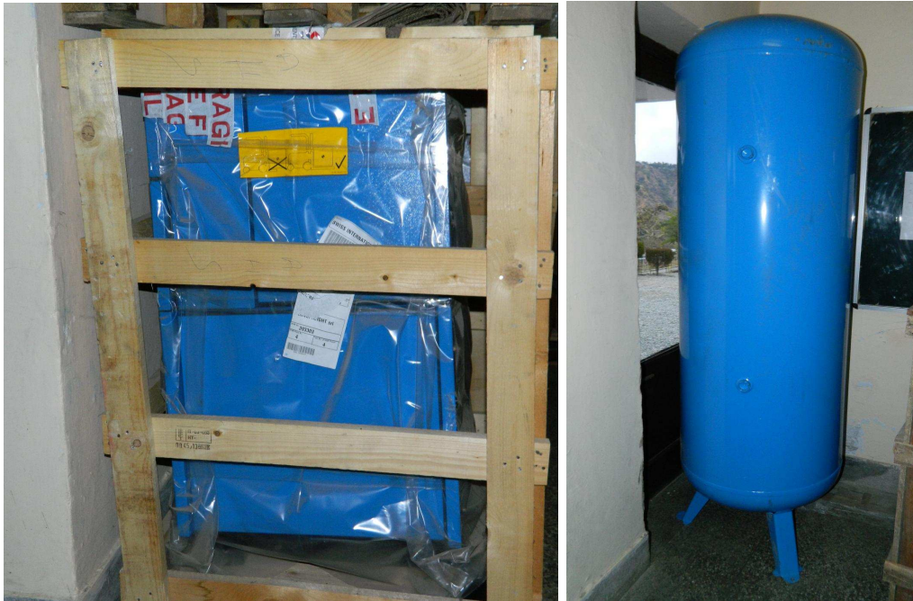
Figure 5.10: Air compressor (left panel) and air receiver (right panel) kept inside the storage room.
